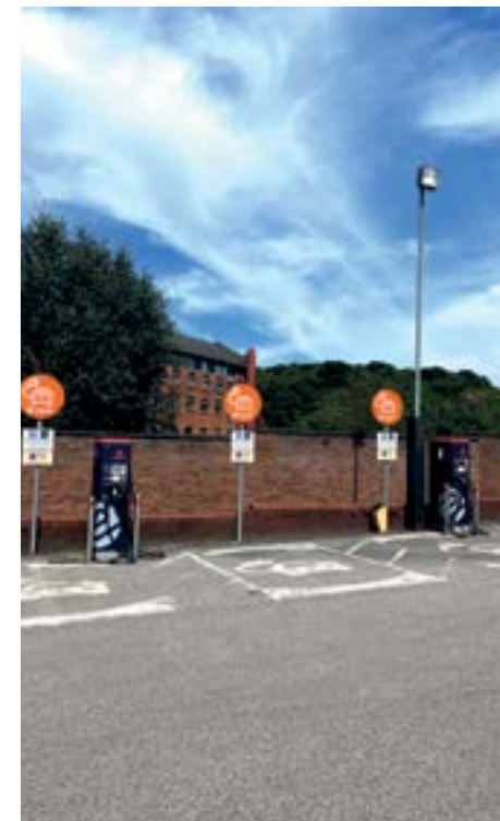
Image above: Electrical Charging Points.
