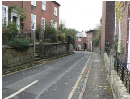
Poor Quality Tarmac Street Surfaces
